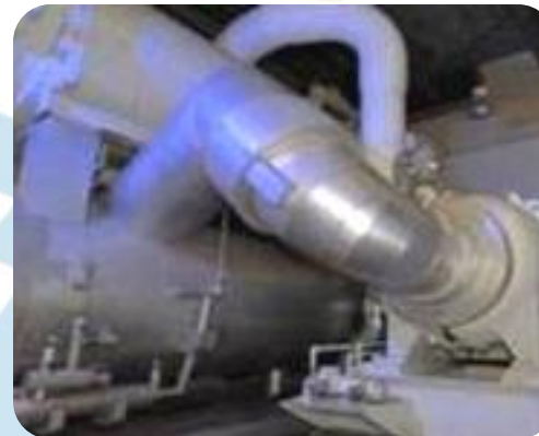
Reconfiguring air-conditioning systems
