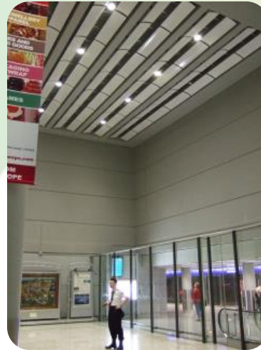
Installations of LED lightings
