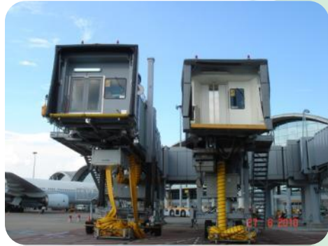
Upgrade FGP & PCA and replace refrigerants
