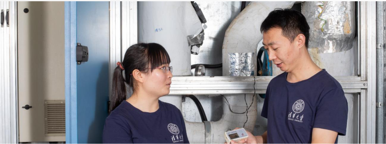
MBCx & Collaboration with Tsinghua University since 2016, identified ~19M kWh savings
