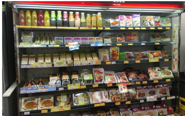
Refrigerator without door 1
